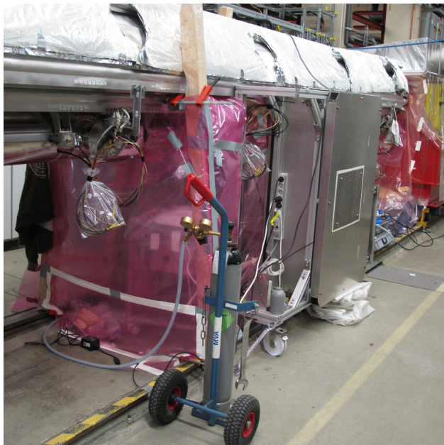
Figure 6: Local clean room at XM22 hanging at the cantilever for HOM antenna exchange.
