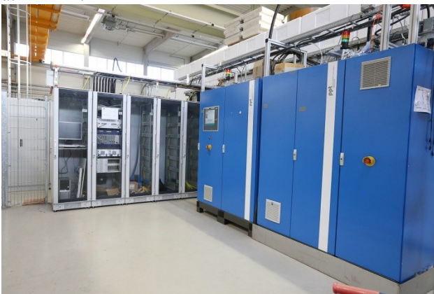
Figure 3: LLRF racks (left) and the 3.9 GHz klystron and modulator racks in the XATB1 module test cave.
